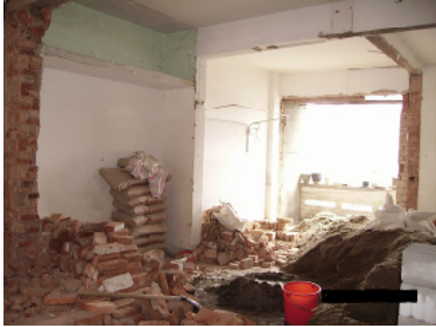
Illustration 2.5 Collapsed walls, which should be marked with safety signs and protective barricades, as in illustration 2.4.
